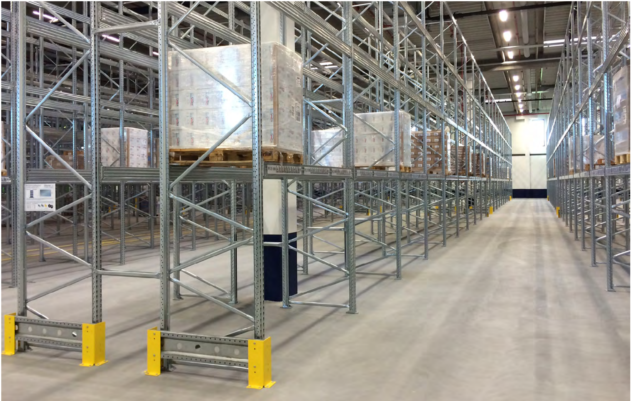
SUPERBUILD - Pallet Racking Reference Installation - Pharmaceutical Products.
